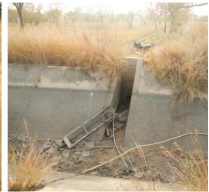
Plate 3: Broken Lateral Gates in Tono Irrigation Scheme
