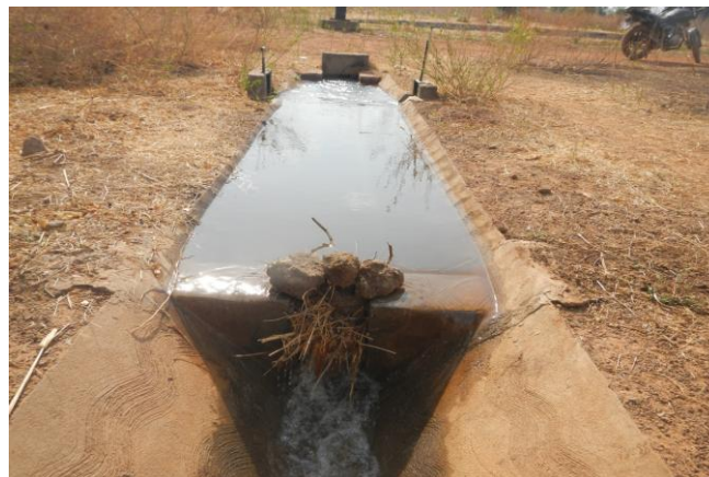
Plate 10: Improvised Lateral Check Structure from Stones and Grass at Golinga Irrigation Scheme
