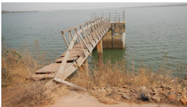
Plate 6: Condition of Walk-Way to Off-take Valves in Vea
