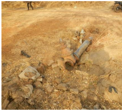
Plate 2: Exposed and Broken Lateral Pipes in Tono Scheme
