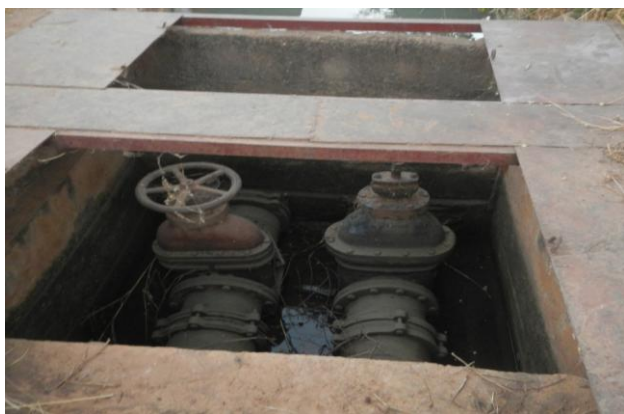
Plate 5: Defunct Off-take Valves in Vea
