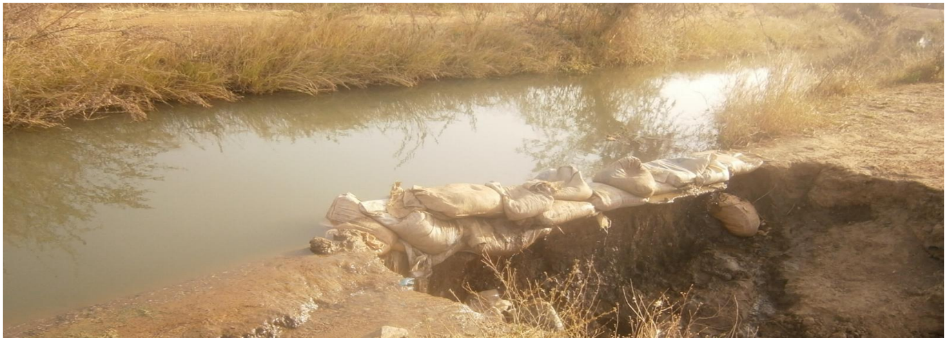
Plate 8: Breached Canal Temporarily Repaired With Sandbags by Farmers in Veia Irrigation Scheme
