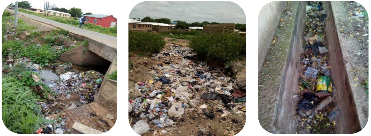
Plate 4.2, 4.3 and 4.4: Show drains choked with solid waste in the municipality
