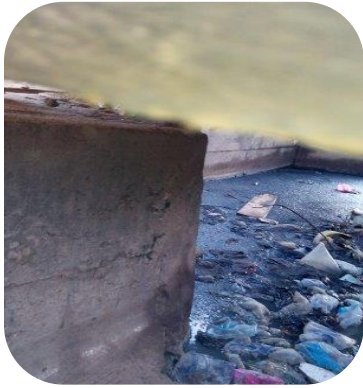
Plate 4.13: Breeding ground of vectors in a chocked and stinky gutter
