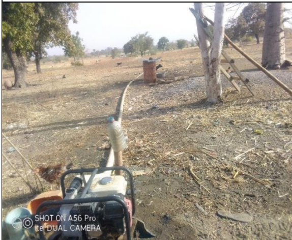
C - Petrol pump abstracting groundwater
