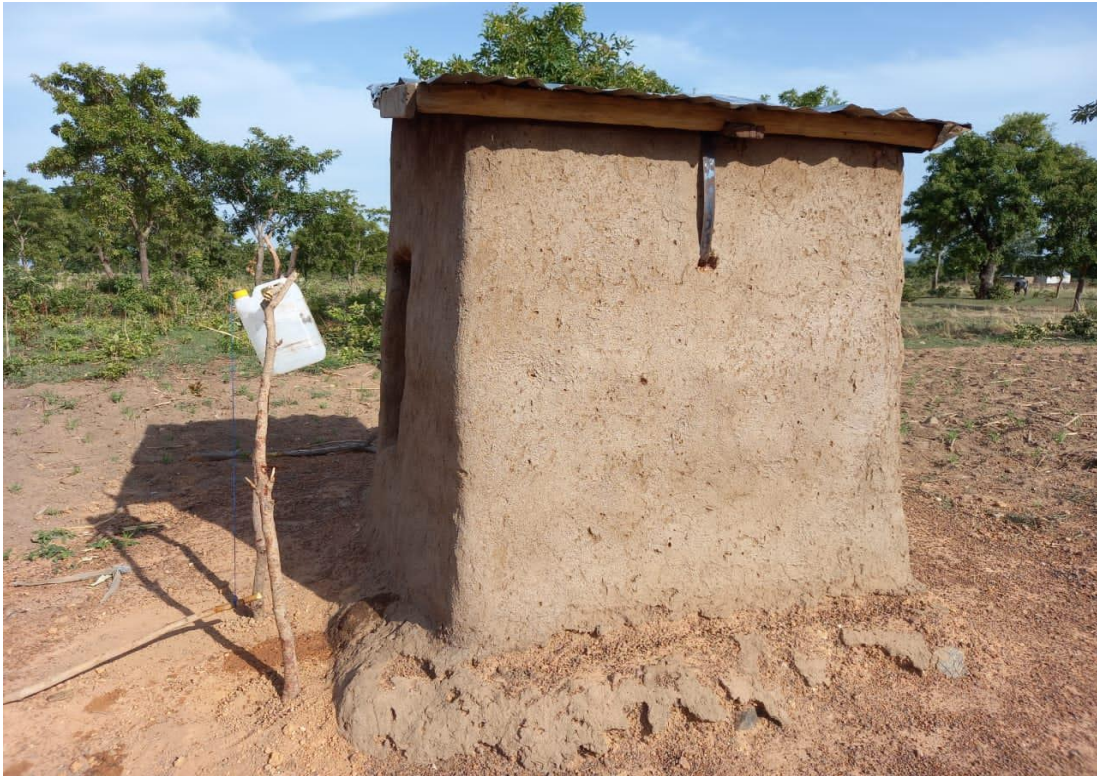
Plate 2: The use of local and some improved materials for household latrine construction with tippy-tap for handwashing.
