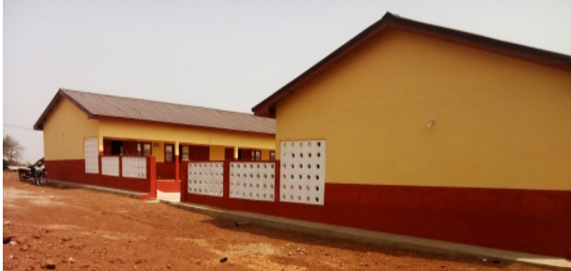
Ongoing 3-Unit Class Room Block With Office And Store And Two Open Urinals At St. Charles Lwanga R/C Primary Malshegu
