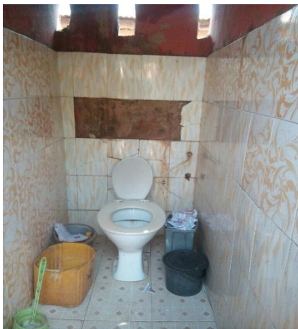
A WC household toilet Facility in Worizehi
