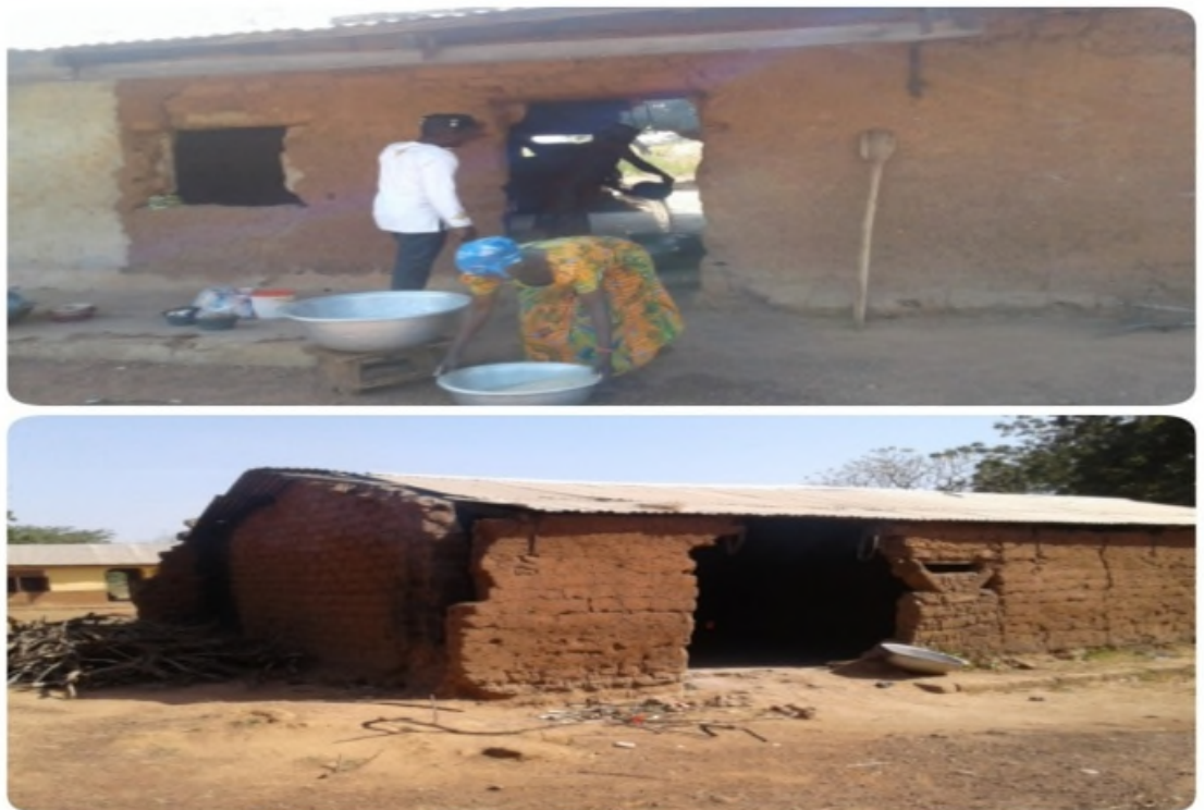
Plate 2.0: Charikpong-Gabilee Basic School kitchen in a deplorable state.
