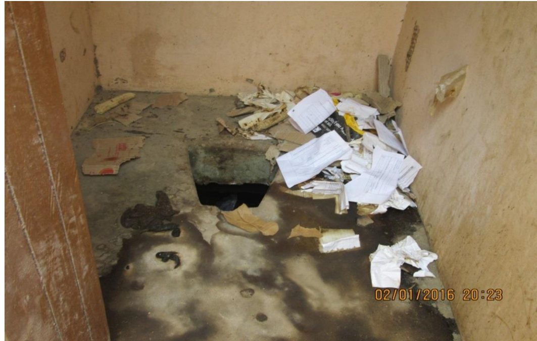
Plate 4.1: Bad state of public toilet at Piisi Market
