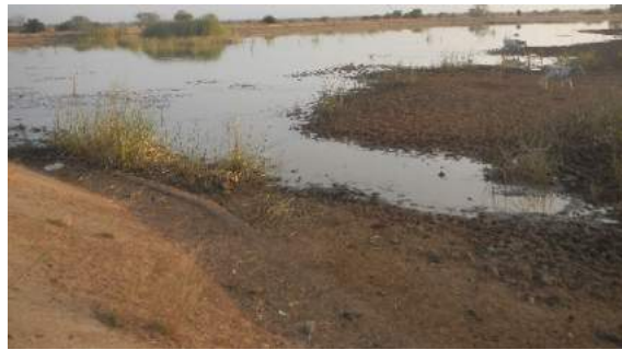
Plate 2: Silted and Weedy Night Storage Reservoir 2 in Tono
