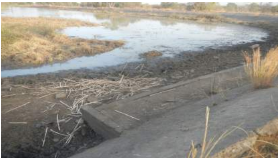
Plate 1: Silted and Weedy Night Storage Reservoir 1 in Tono
