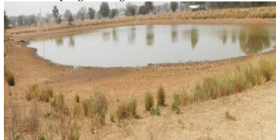
Plate 6: Silted Night Storage Reservoir in Vea Scheme
