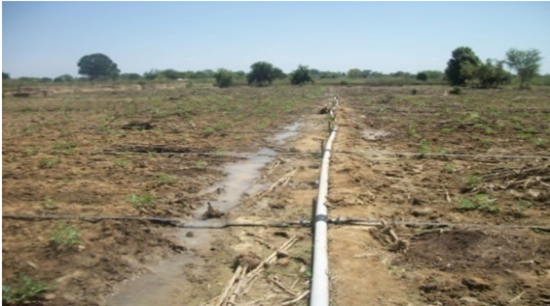
Plate 4.8 Drip lines connected to a Main line on field
