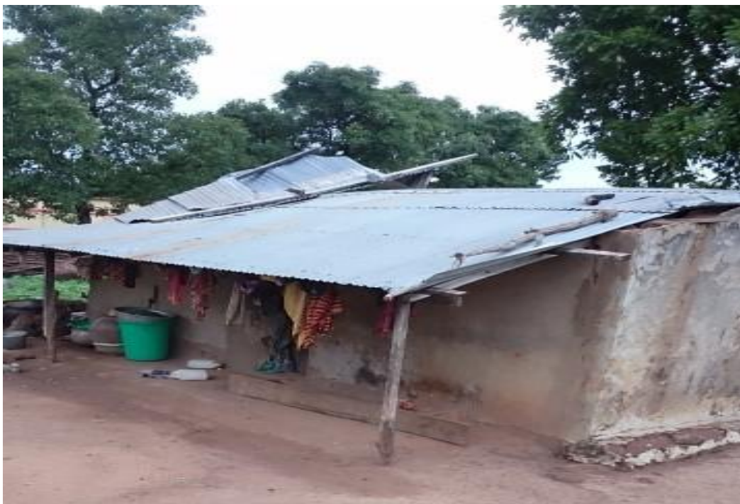
Figure 3. Picture depicting a house affected by rainstorm (Source: Fieldwork, 2014)
