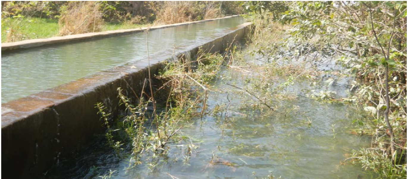
Plate 3.2: Spillage from Canal Causing Waterlogging in the Veja Irrigation Scheme
