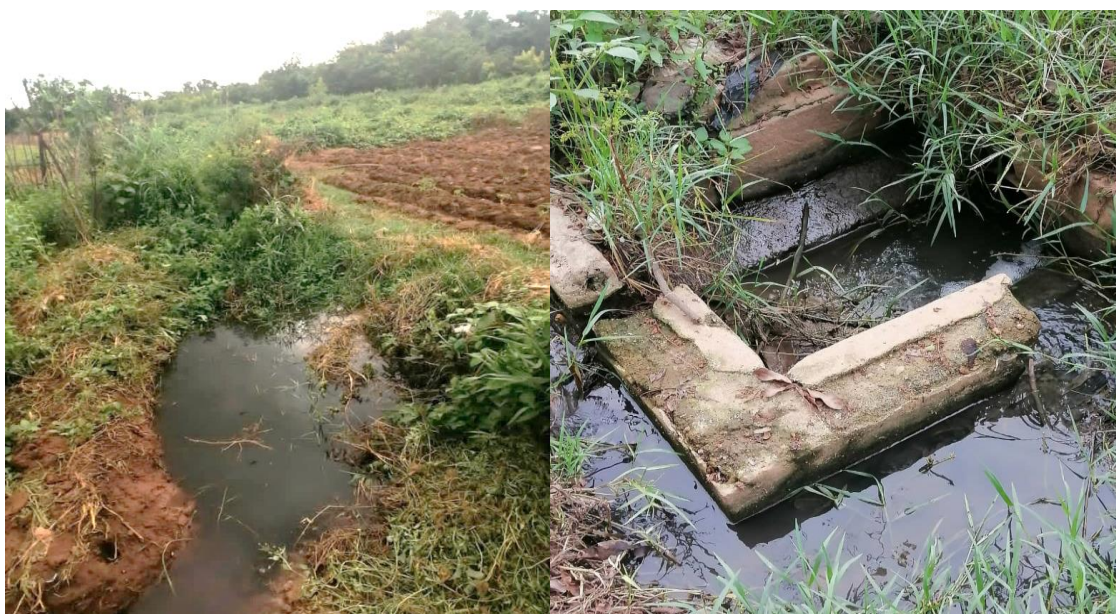
Figure 2: Domestic Wastewater at Zagyuri flowing from Kamina Barracks
