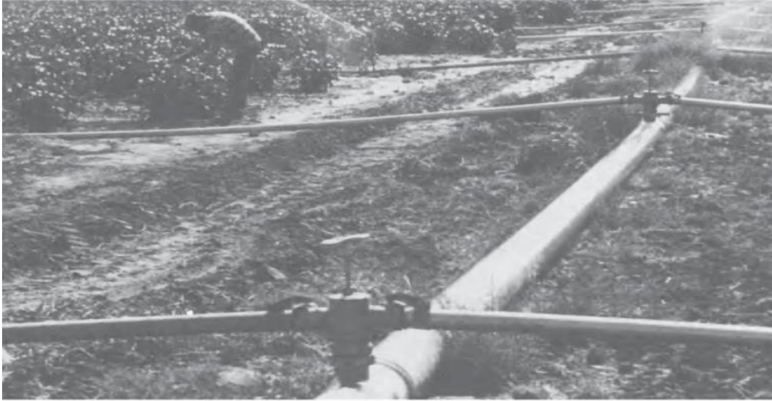
Plate2. 7: Solid-Set Sprinkler Laterals Connected to Portable Aluminum Mainline.
