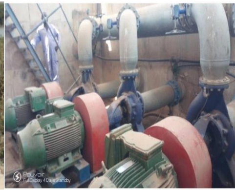
Plate3. 3: Pumps and Power Unit
