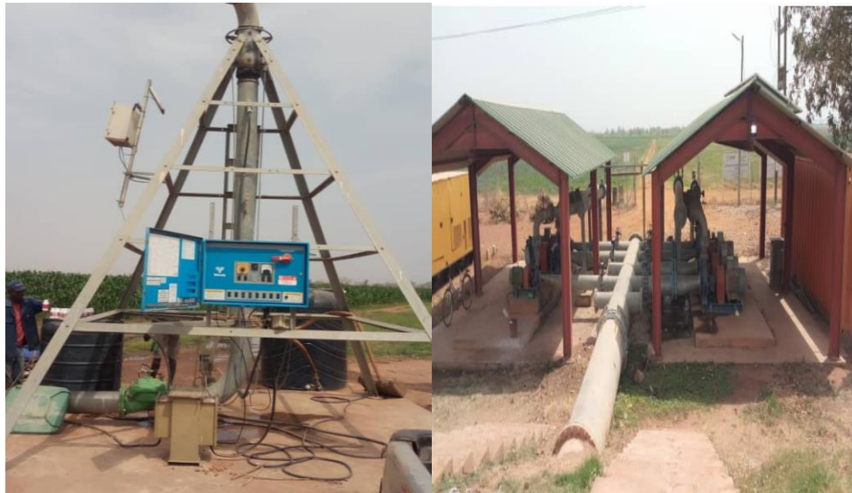
Plate3. 10: Control Panels and Pivot Point
