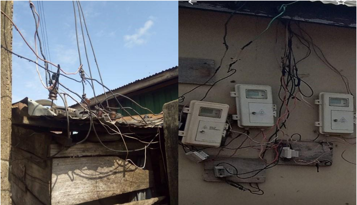
Plate 4.1a and 4.1b Electrical connection in Aboabo and New Jisonayili
