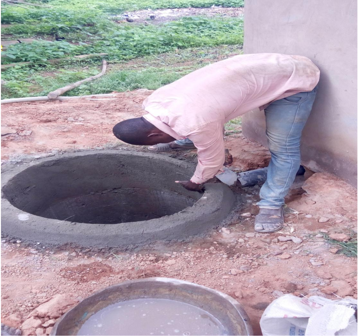
Photo of a Construction of a Latrine after the implementation of CLTS Approach
