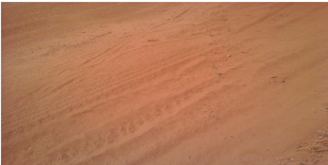
Image 4.6: A Road Destroyed by Heavy Tipper Trucks Plyng the Roads to the Gravel Pits
